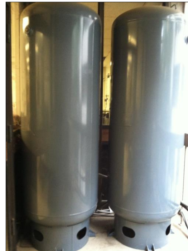
MP tanks on balcony
